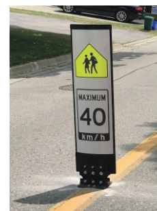
One of 3 new speed posts on Romfield Circuit
